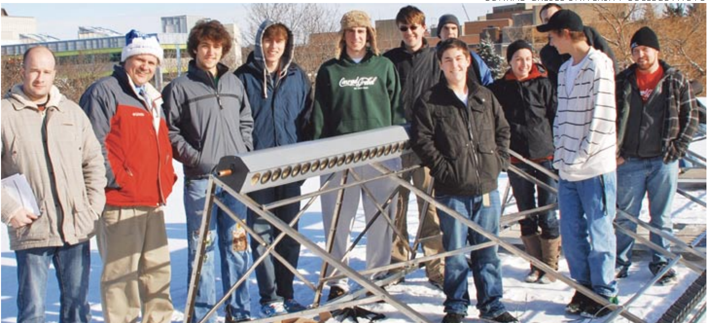
Solar Grebel students are thrilled to watch their green dreams take shape as they stand on the roof at Conrad Grebel University College with a partially installed solar thermal collector.
