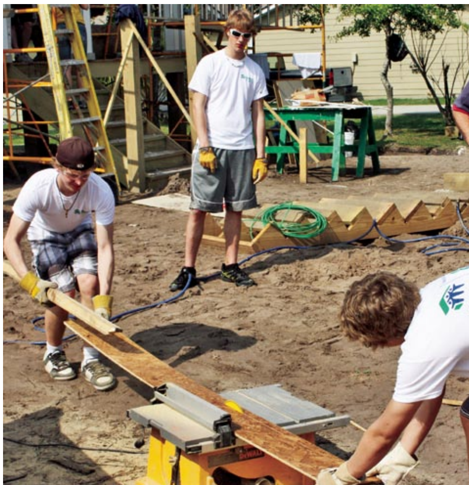
Every year, Rosthern Junior College staff and students from Saskatchewan partner with Habitat for Humanity to assist in the construction of homes for needy families.
