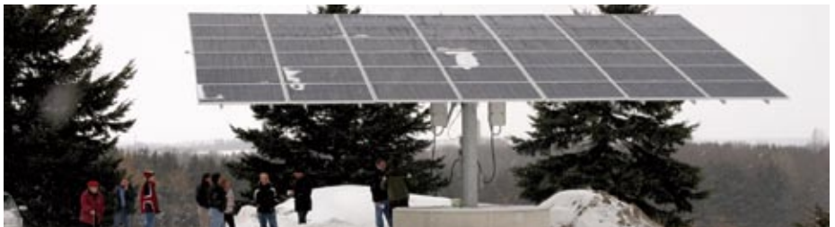
Solar electric panels at Hillcrest Mennonite Church, New Hamburg, Ont. (2011).
