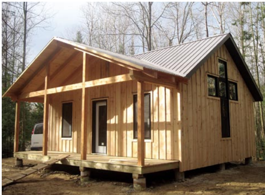
Two new camper cabins were constructed at Silver Lake Mennonite Camp as part of a half-million-dollar capital project. Both are insulated for year-round use.
