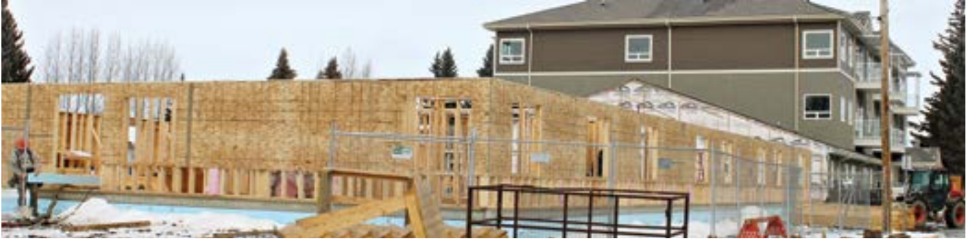
Phase 2 of the Prairie Meadow Place construction project will add another eight single- and four double-rooms to the assisted living facility.
