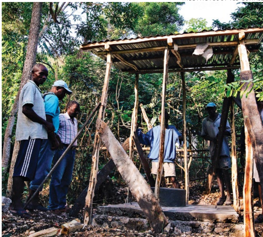
This is the frame of the first latrine to be built as part of MCC’s project in the rural community of Wopisa-Gabriyèl in Haiti.
