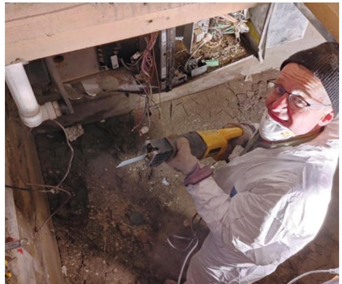
Tim Kuepfer spent half a day in a crawl space, disconnecting and removing a furnace destroyed by the water and muck.
