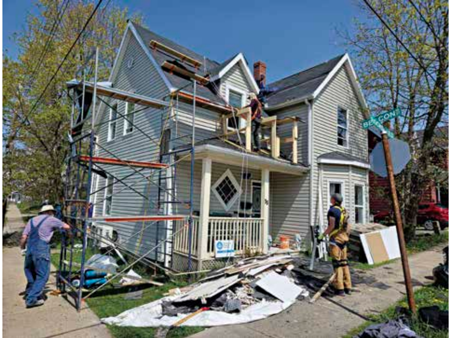
Volunteers work on repairing the roof of a hurricane-damaged home on Cape Breton Island.
